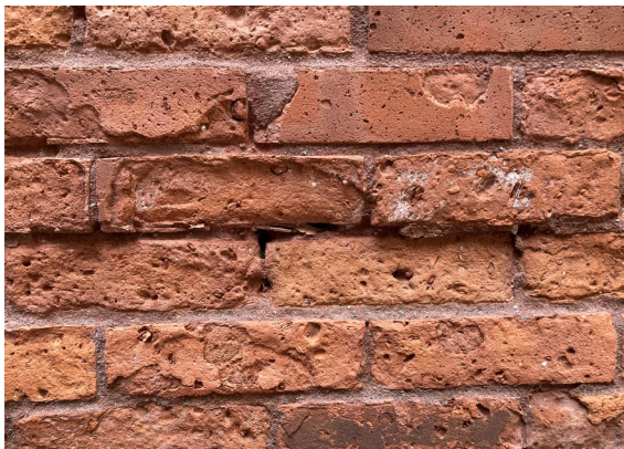
Pictured right: detail of crumbling bricks and missing mortar; detail of relatively new bricks (on south side of Central, new, accessible entrance built 2015)
